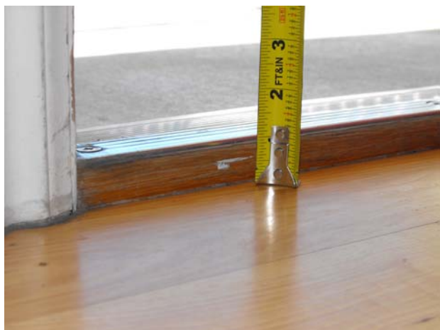
Door sills/thresholds should be level. A sill even an inch in height is a significant trip hazard for even the most able bodied person.
